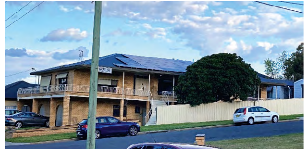
17KW Solar PV System installed at Broughton House, Albury by Straight Line Solar.
